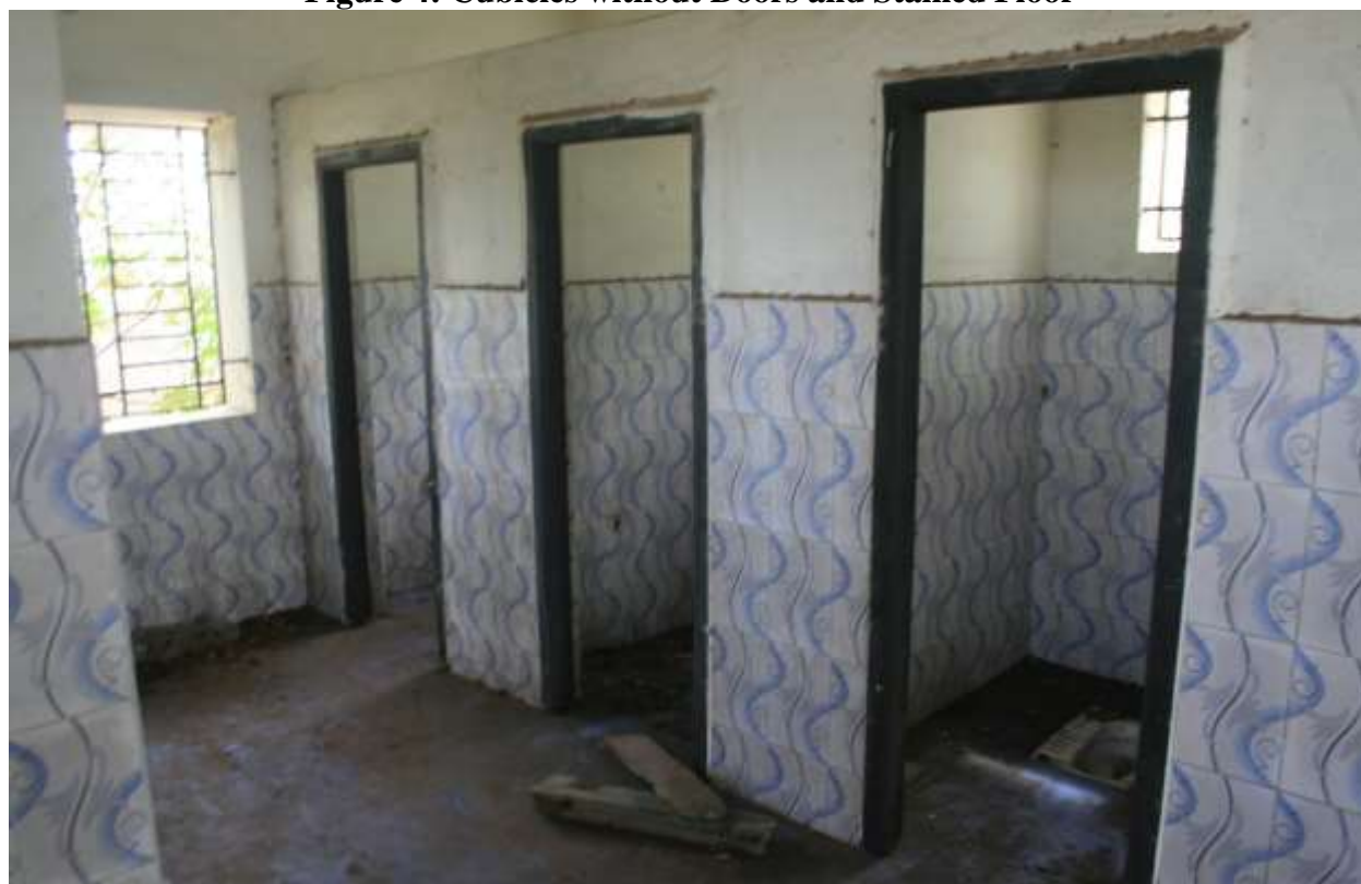
Figure 4: Cubicles without Doors and Stained Floor
