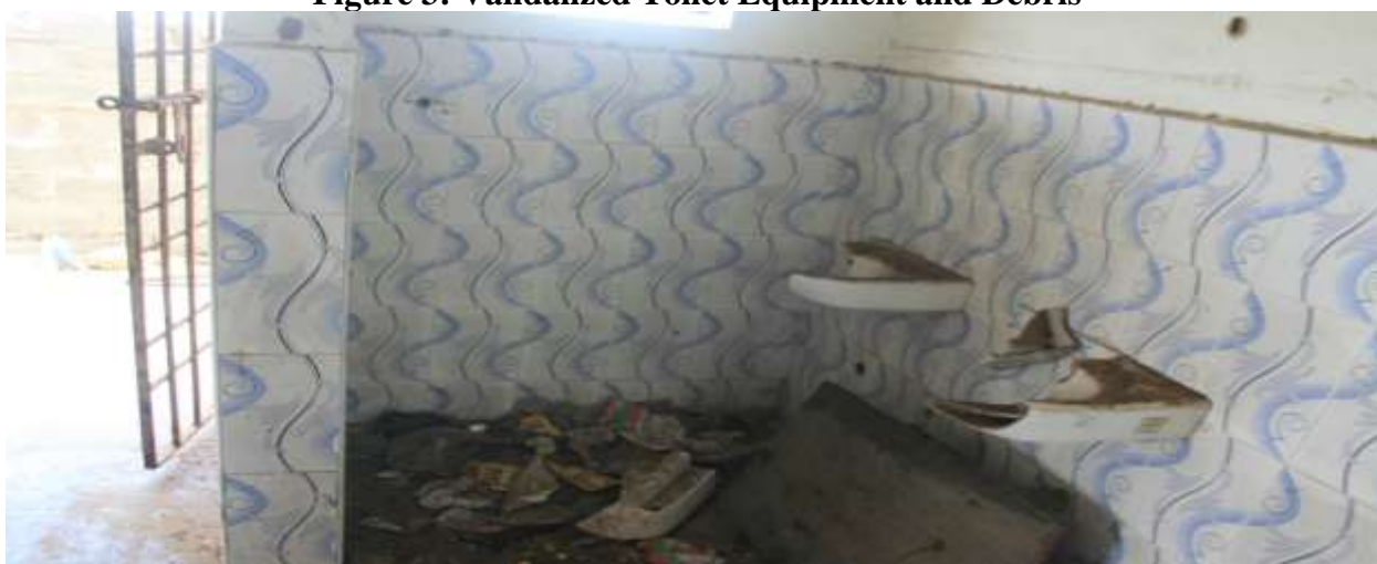
Figure 3: Vandalized Toilet Equipment and Debris
