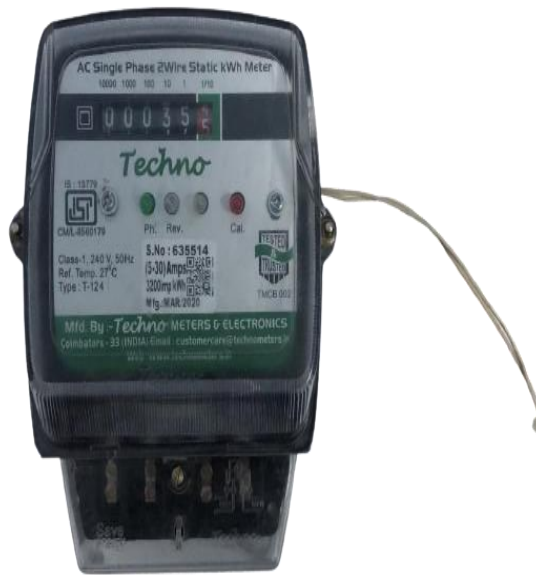
Figure 2. Energy Meter After Tapping
