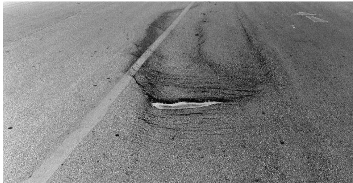
Figure of slippage failure
