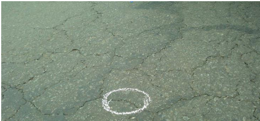
Fig. 2 Alligator map cracking at Km 45.30 Chennai-Tada road, N.H.5
