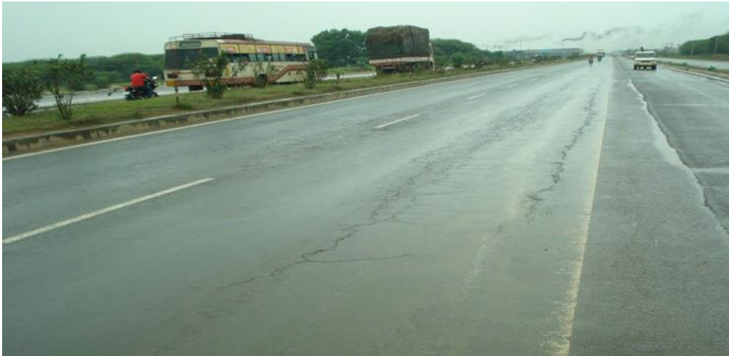
Fig. 4 Longitudinal cracks at Km 36 Chennai-Tada road, N.H.5
