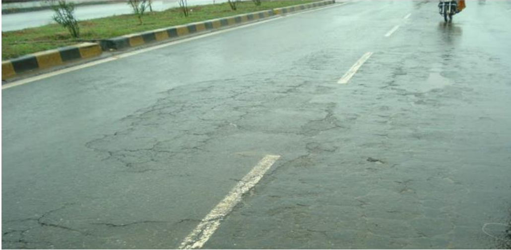
Fig. 3 Severe map and block cracking at Km 32.350 Chennai-Tada road, N.H.5
