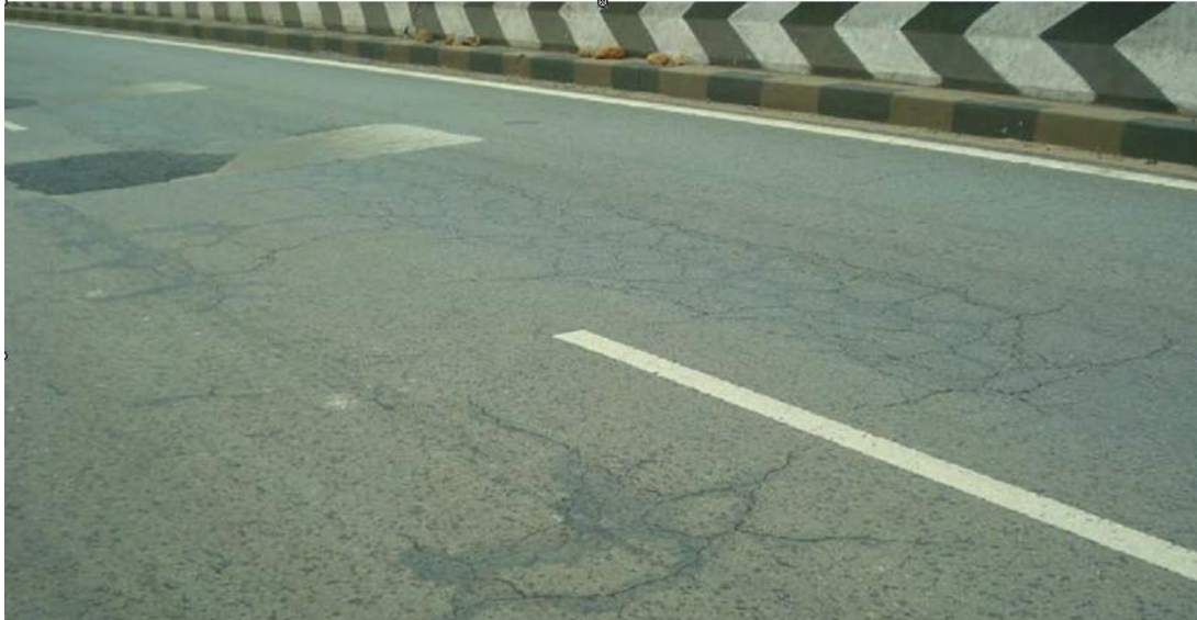
Fig. 1 rutting and cracking along wheel path at Km 53.00 Chennai-Tada road, N.H.5
