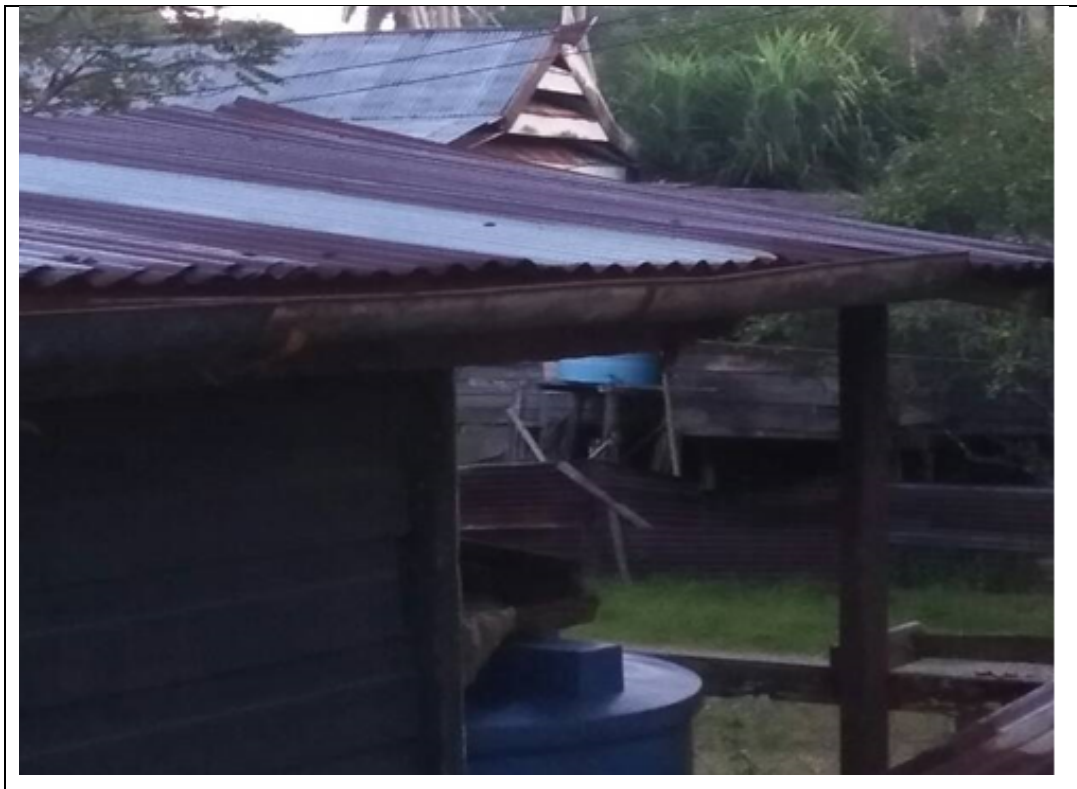
Figure 6 House roof that has been oxidised used as a storage device for the use of RHS in Kg. Wallace Bay
