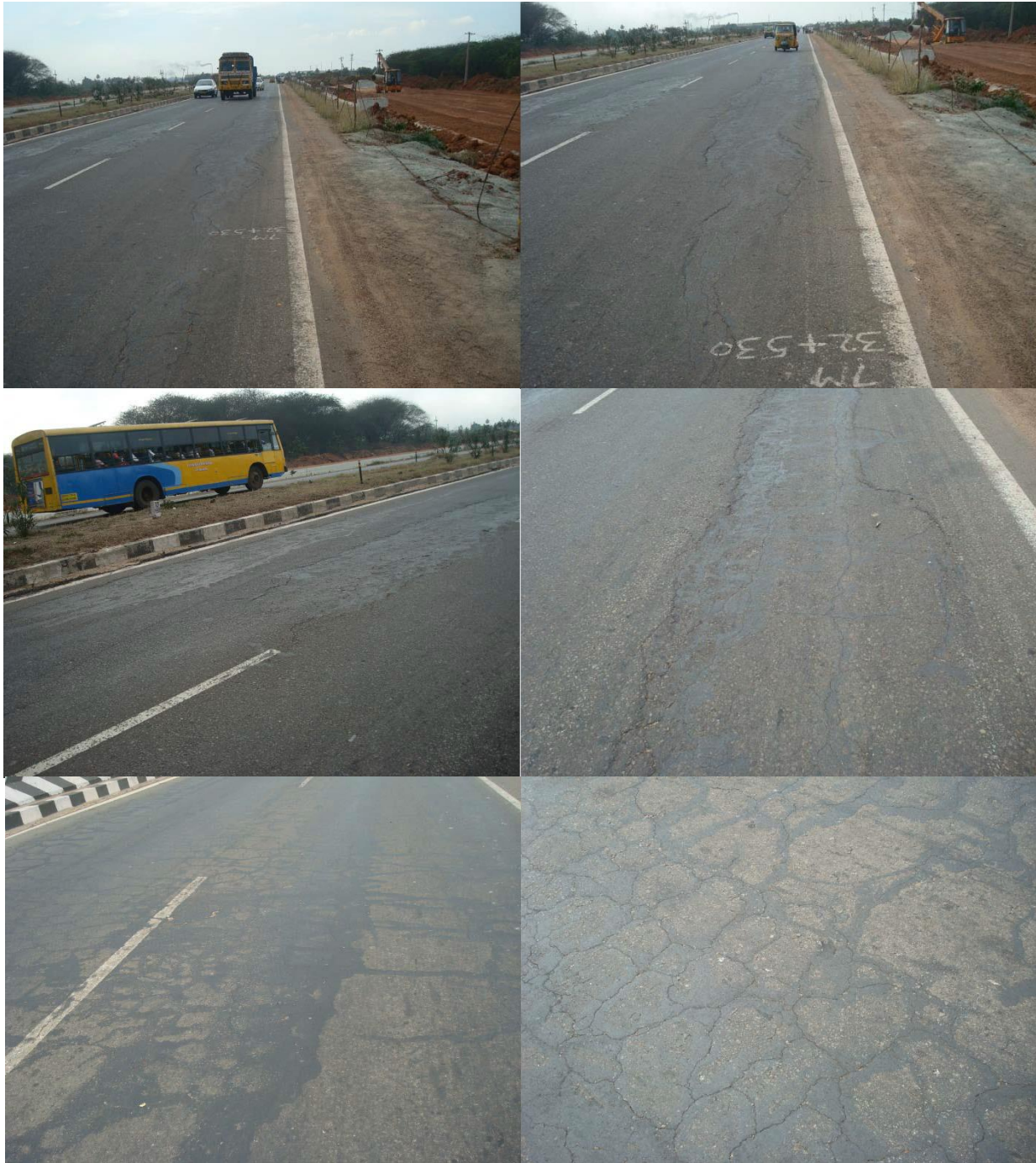
Figure 2: Severe wheel path fatigues cracking, rutting, shoving, and inadequate cross slope Chennai-Tada Road NH-5.
