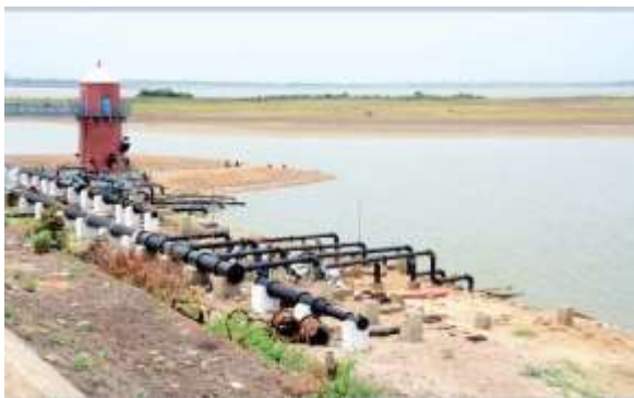
Fig.5 Red Hills Reservoir in Monsoon failure when scarce water is pumped into the otherwise gravity intake.
