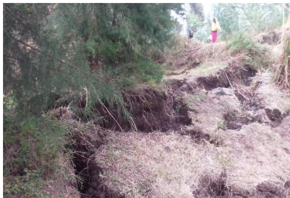
Fig. 6. Large Tension cracks appeared in earth slope failure
